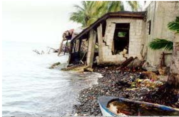
Erosion placing homes at risk in St. Margaret's Bay
