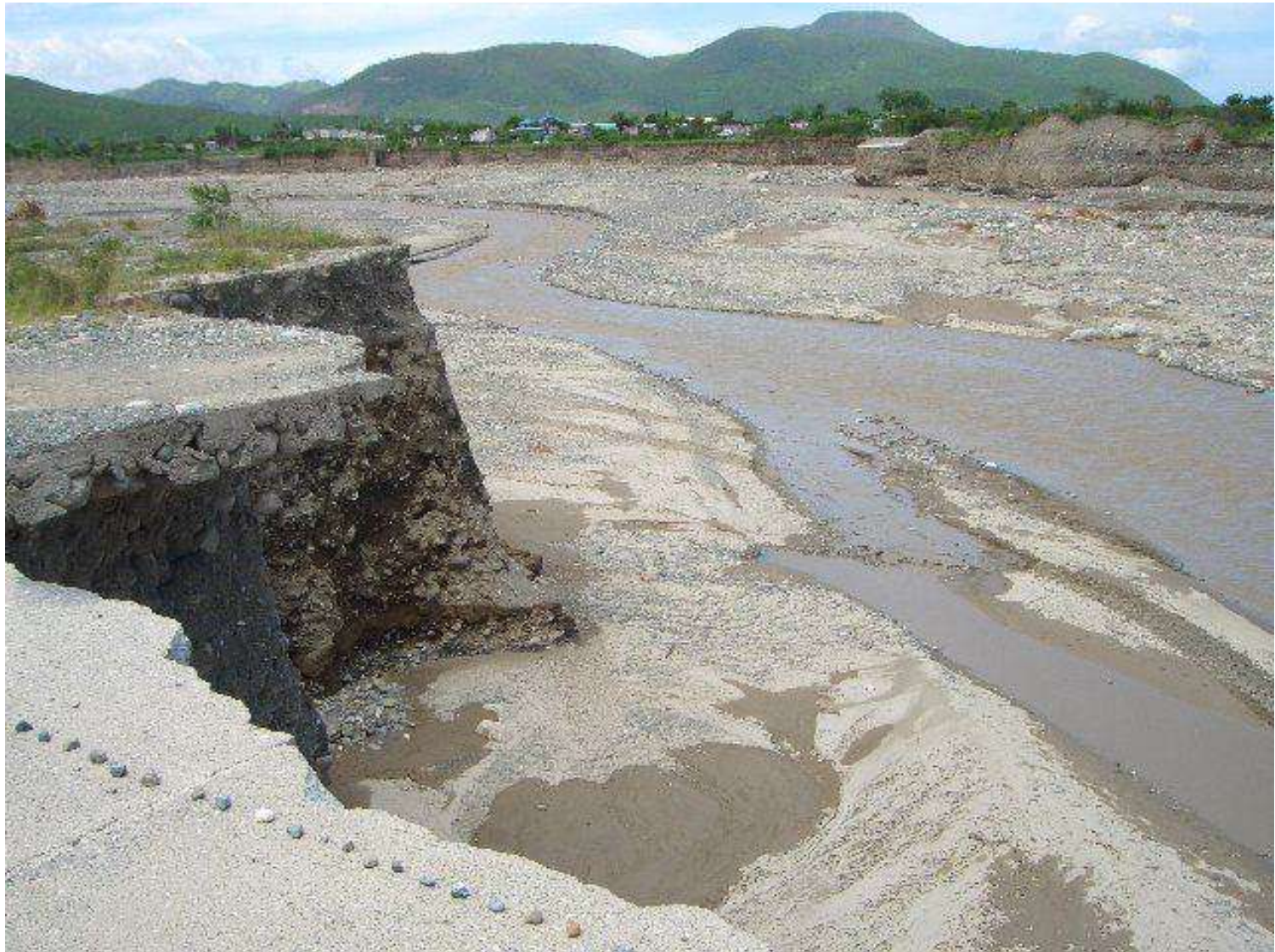
The destroyed bridge at Harbour View, St Thomas following Tropical Storm Gustav, 2008
