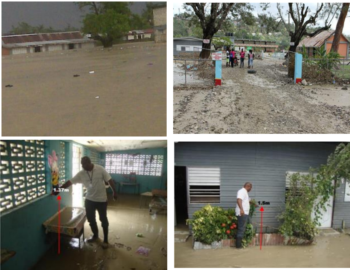
Figure 5 Flooding at Port Maria Primary (top) and Secondary (bottom) Schools, 2012
