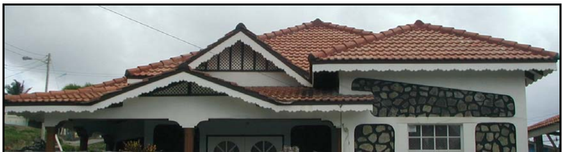
Figure 4.2: Another type and very uncommon roofing tiles in St Vincent, note the more common corrugated sheets shown in fig 4.1
