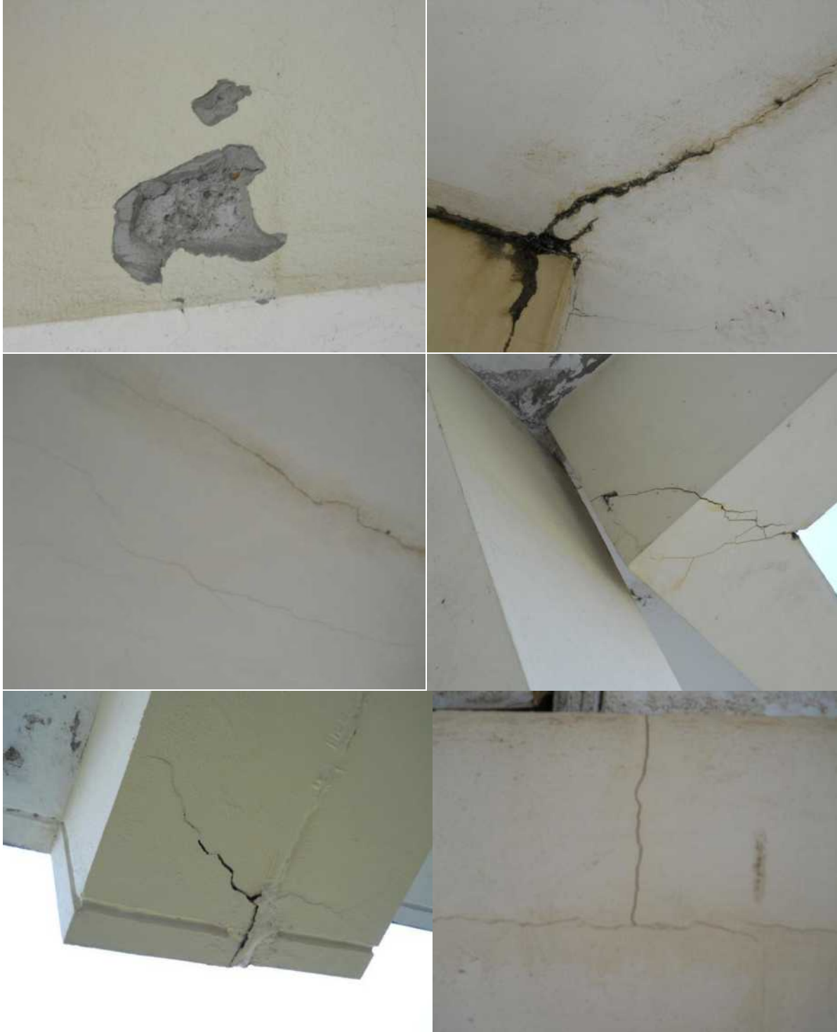
Figure A2: A group of pictures showing major defects to the Annotto Bay High School, in the form of major cracks in vital structural members (Beam) and also pop-outs. There is also evidence of water contact which suggests that reinforcements are being damaged (rust) which cause swelling of the bars, which reflect pop-outs and cracks.
