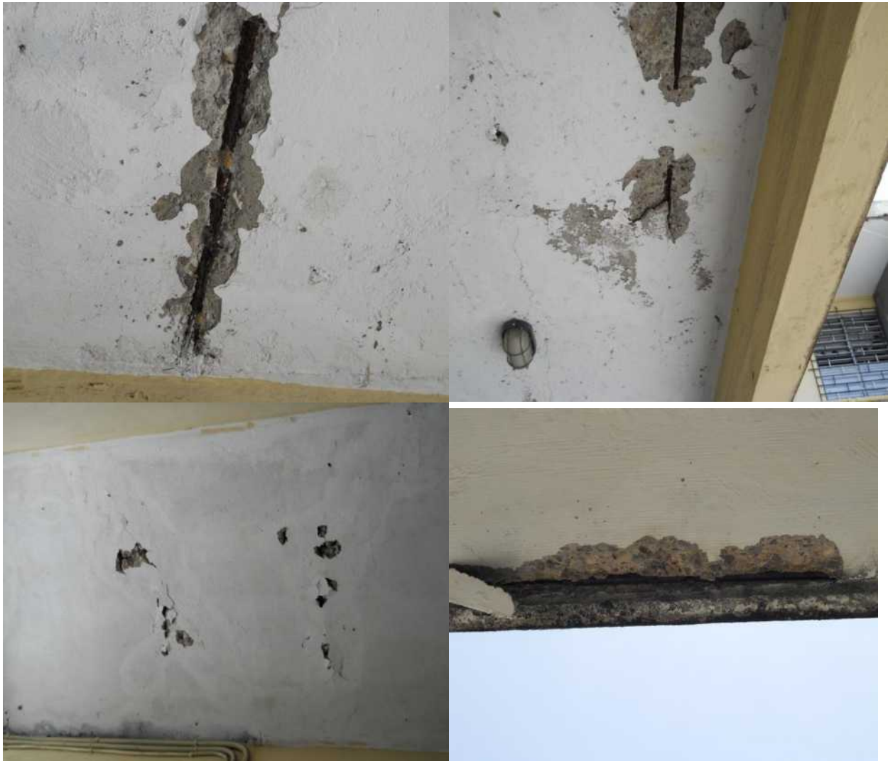
Figure A1: A group of pictures showing major defects to the Annotto Bay All-Age School, in the form of pop-outs and exposed reinforcement. Due to the exposure of these bars they have begun to rust and over-time will increase the risk of failure.
