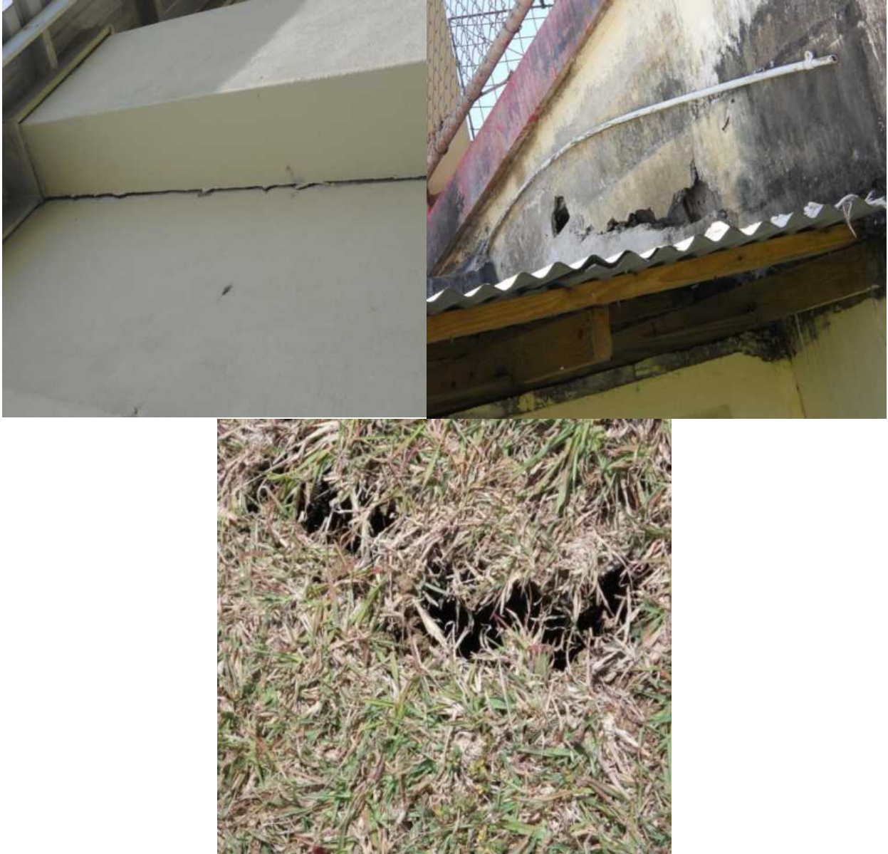
Figure A3: A group of pictures showing defects to the Annotto Bay Hospital in the form of major cracks and the moving away of a column from the building due to the presence of soil movement, which actually left large cracks in the ground.
