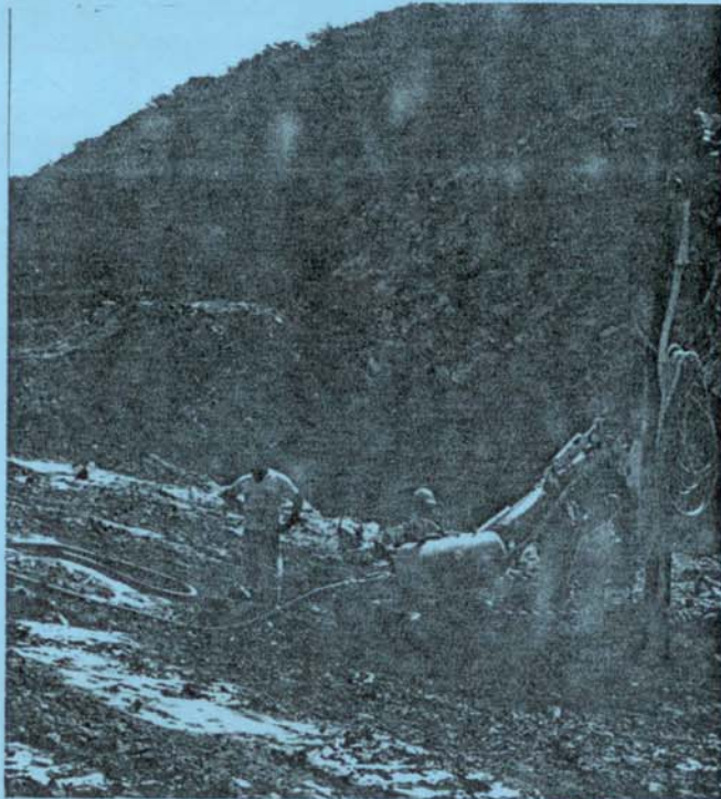
Production Drilling, Northwest of the Bito Quarry at The Jamaica Gypsum and Quarries Limited (JGQ).
