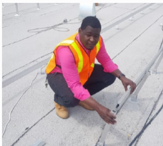
Dudley Williams, Postgraduate Physics Student, Faculty of Science & Technology, The UWI, Mona, assisting with the installation of the racking system and clamping of the electrical wires on the roof of the Physics Building
