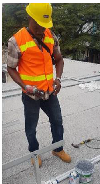
Leaford Henderson, Postgraduate Physics Student, Faculty of Science & Technology, The UWI, Mona, on the roof of the Physics Lab, preparing and using the impactor drill to screw the clamp which holds down the PVC pipe for the electrical cables
