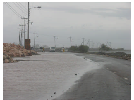
The Palisadoes road looking west, washed over, but not impassable
