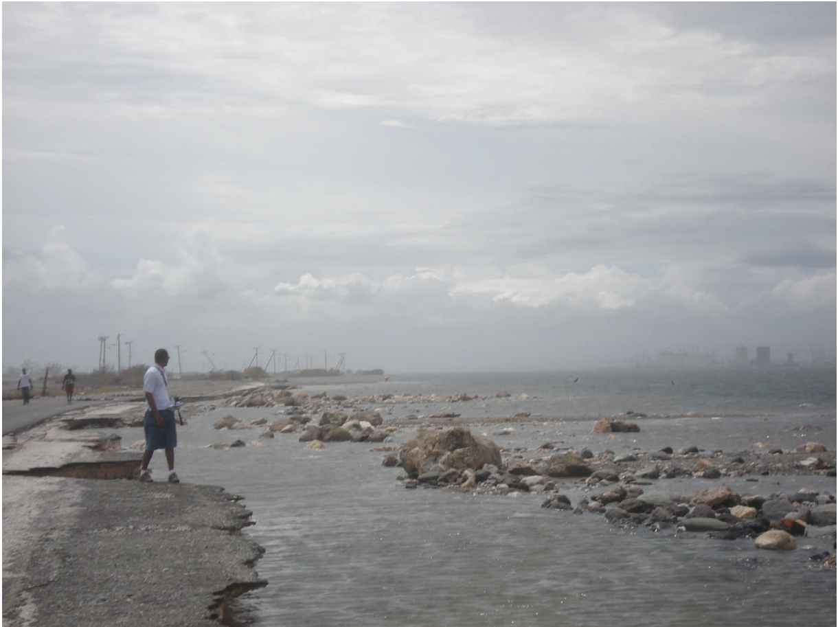
1) Photo of a section of the road badly damaged during Hurricane Dean
